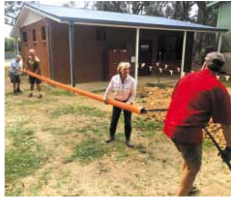
Chris Chambeyron, Merv Hooper, Tracey Martin and Glenn Davies laying the cable
