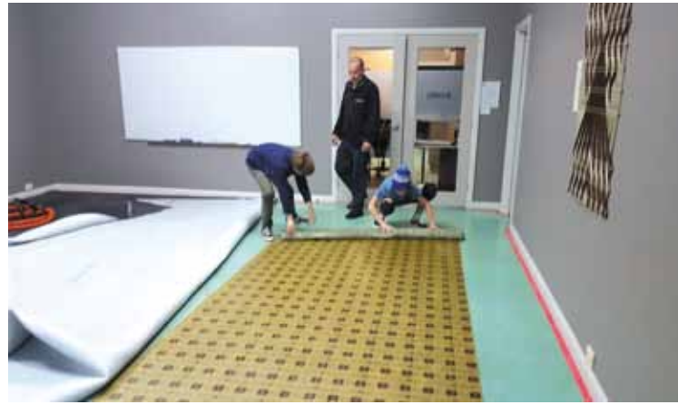
Jasper, Duane Washington from Sommers Flooring Xtra and Will removing carpet and underlay from the Board Room
