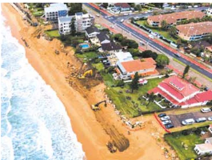
Collaroy beach - desperate attempts at erosion repairs Photo Credit: Getty
