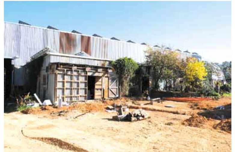
Site preparation at the Agency of Sculpture for the Yack01 community-scale battery, with the solar panel arrays just visible along the roofline. Photo: J Milbank
