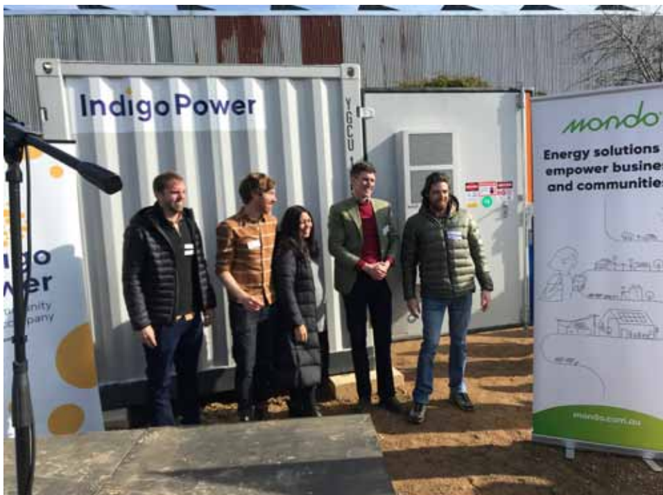
The Indigo Power Team standing in front of the battery unit
