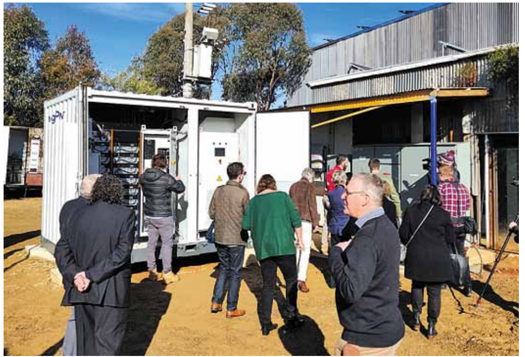
About 180 people attended the launch at the Agency of Sculpture and checked out the 274 kWh battery and switchboard. Photo Credit: J Millbank
