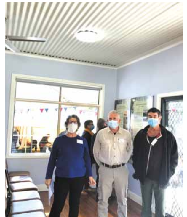
From left to right: Bruarong Hall committee member Ruth Yule, YCDCo Board Member Max Horvath and Dan Carberry of Classical Constructions admire the new acoustic ceiling at the launch of the Bruarong Capturing History Project from beneath the pesky masks
