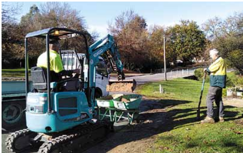
Work under way to resurface paths at the Community garden by contractors and members. PC: David Thorpe
