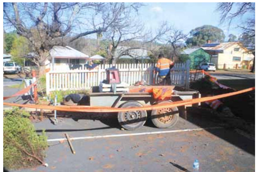
Trenching works start in the car park at the rear of the Senior Citz.
