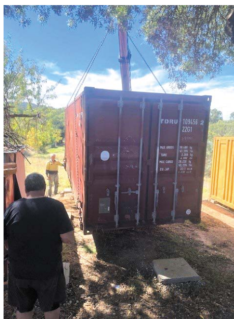
The new storage container being expertly lowered into place at the Yack Shack. PC: Graeme Neil
