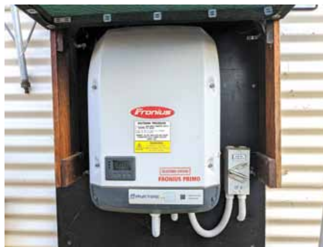
The solar panels inverter
