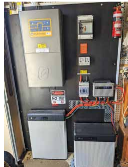
Batteries and Control Panel
